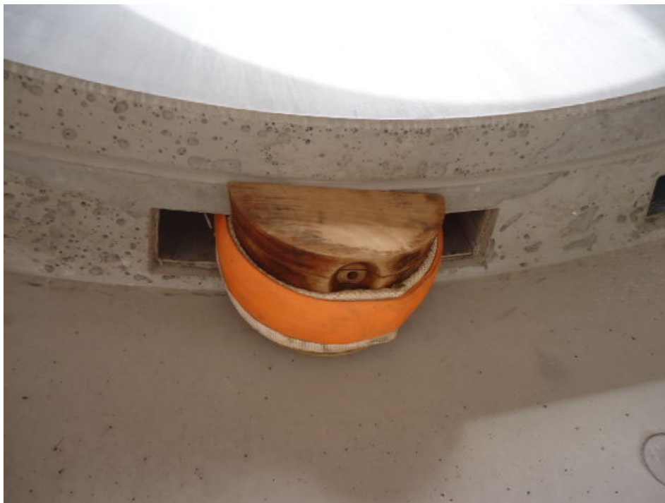
Figure 8: Example for fixation of a slippage around a wooden wedge on the bottom edge of the connection-element
