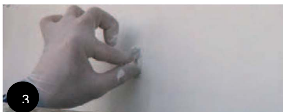
3 Ensure that the facade panel caps are clean and dry before fixing.
