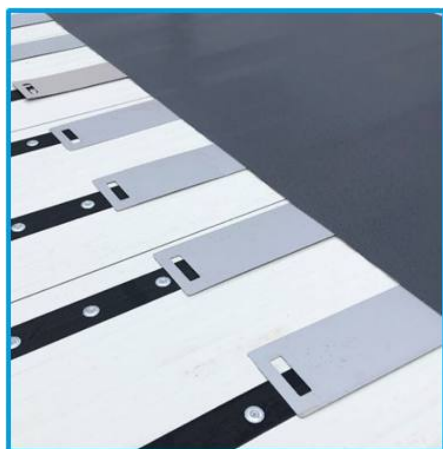
"BMI InnoGrip strips" are temporary protected with "BMI InnoGrip installation sheets" prior to laying the membranes
